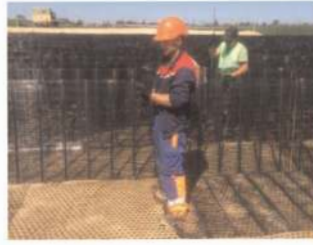
Figure 5. The general view of a geomattress.
