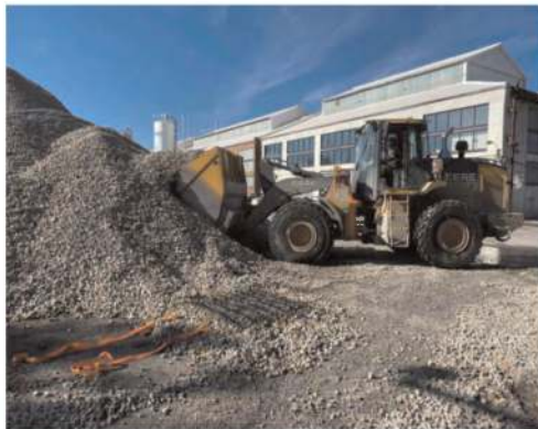
Figure 1. Photograph of UL-FGA installation.
