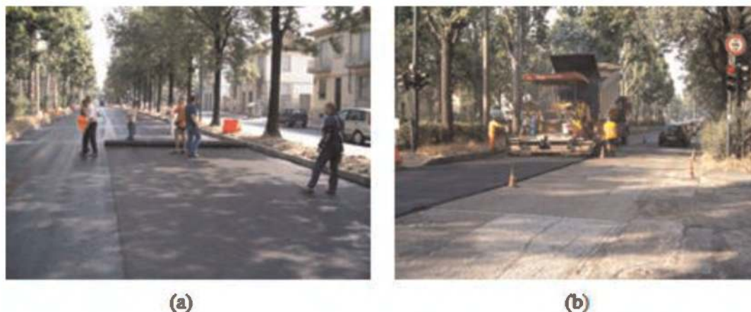
Figure 1. Installation of the HaTelit C 40/17 asphalt reinforcement (a) and asphalt placement on unreinforced section (b) (June 2005).
