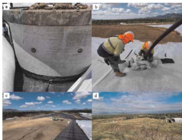
Figure 5. a) BGM to concrete connection, b) BGM to polymer pipe connection, c) photo during construction d) photo of completed cap with vegetation.
