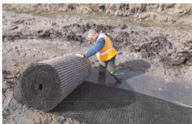
Figure 15. Installation of a reinforced High Performance Turf Reinforcement Mat (HPTRM) for slope protection.
