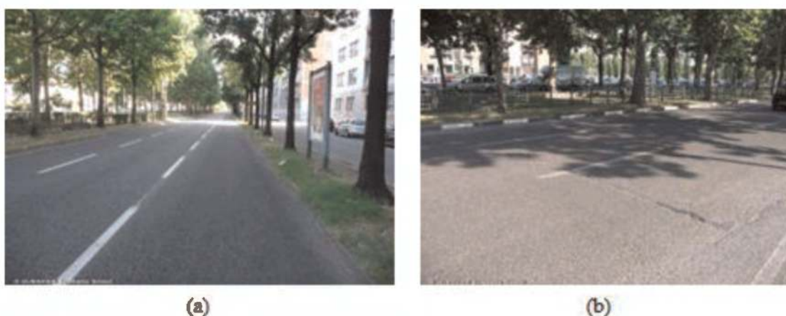
Figure 2. HaTelit C 40/17 reinforced area without cracks (a) and unreinforced section presenting reflective cracking (b) (July 2009).
