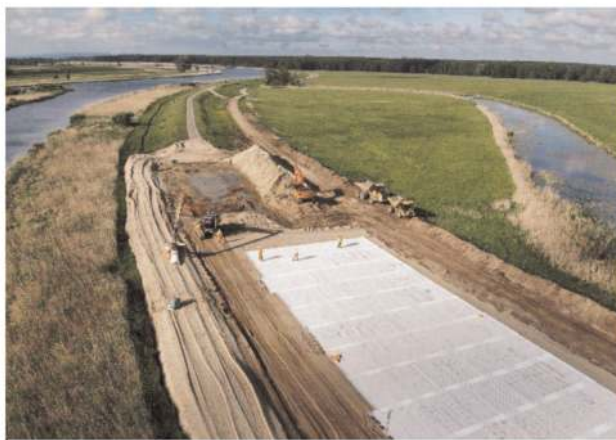
Figure 16. Installation of high strength geogrids as basal reinforcement below the flood defence at the Oder dike, Germany.
