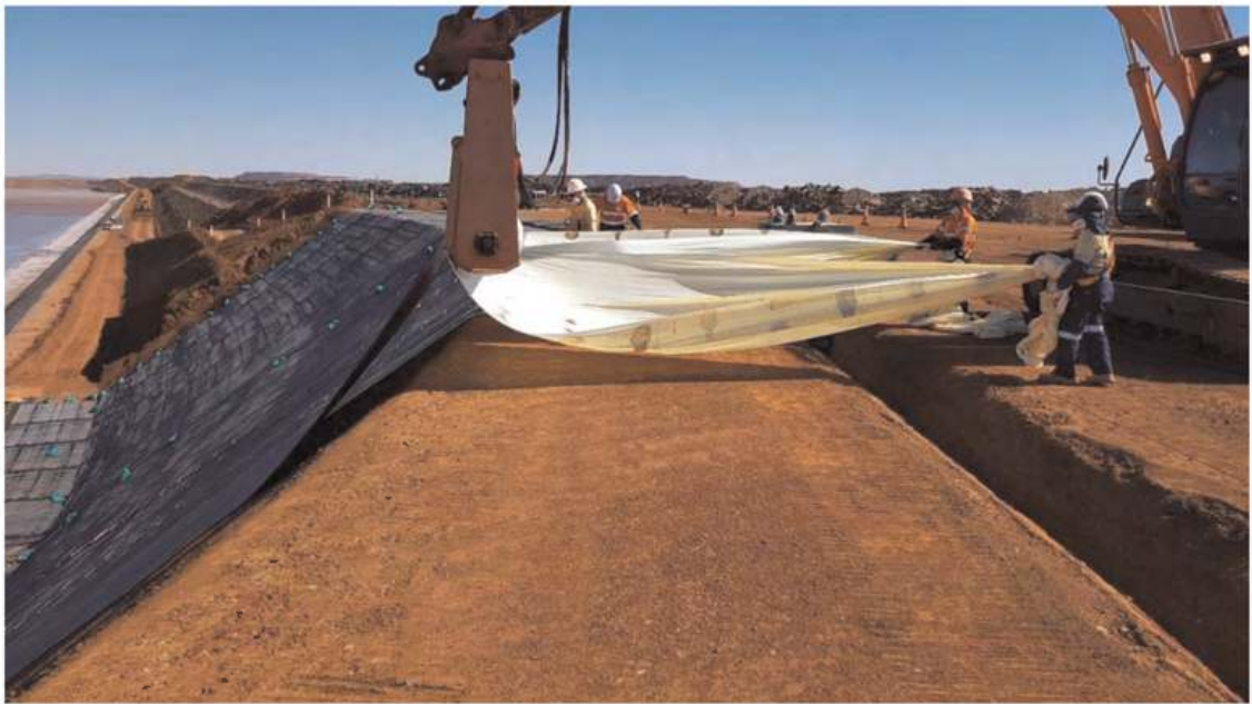
Figure 7. The innovative High Friction Angle BGM being deployed on a steep 1.3H:1V Tailings Storage Facility. The white siliconized layer is removed at time of installation to provide a bitumen surface on the underside which maximizes the interface friction angle with the subgrade. This photo also shows another innovation in terms of safety with regard to geosynthetic installations, with the hydraulically operated deployment beam, which uses hydraulics from the excavator. The hydraulic beam enables a safe and control deployment on these steep slopes and it also helps reduce worker fatigue on extremely hot sites.
