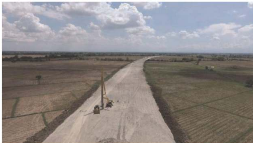
Figure 5. PET high strength geotextile reinforcements laid with principal strength direction across the embankment, followed by placement of gravel layer on top.
