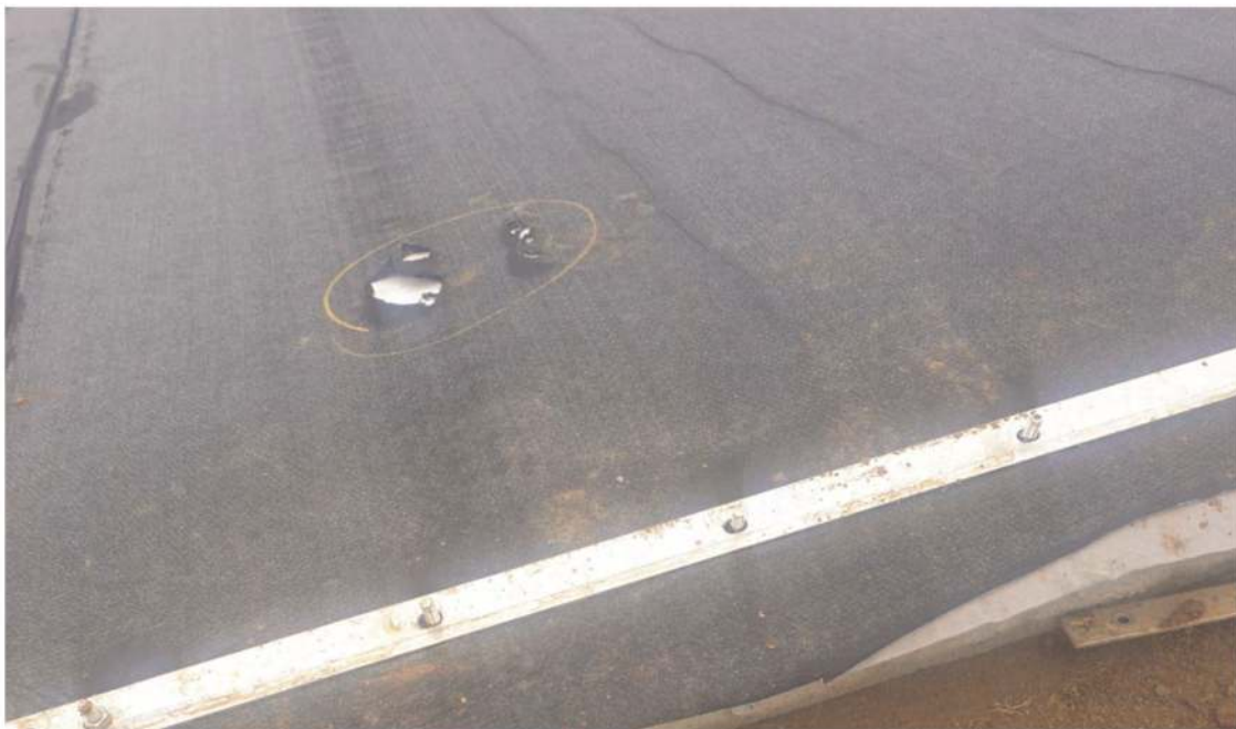
Figure 5. Holes in a conductive composite made by workers walking on it. These required patching to ensure adequate conductivity.
