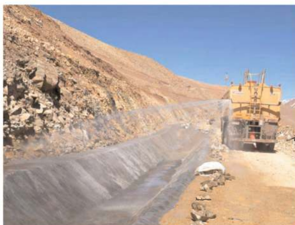
Figure 2. GCCM hydrated by surface spraying resulting in pooling water in the invert. These parts of the GCCM structure cure in immersed conditions.
