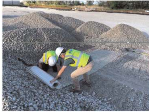
Figure 6. Photograph of PHL Ron installation.
