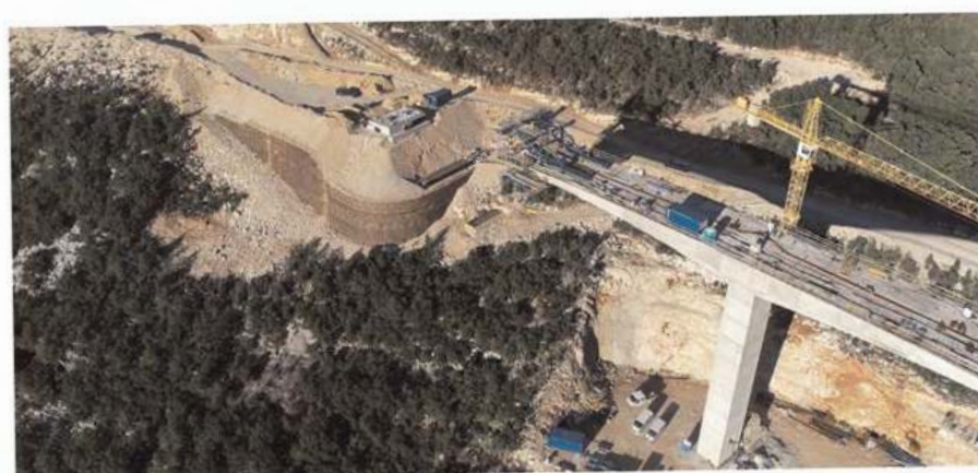
Figure 6. Aerial drone view of the U0 wing wall and abutment of the Dumanja Jaruga viaduct made with the reinforced soil technique with extruded HDPE mono-oriented geogrids.
