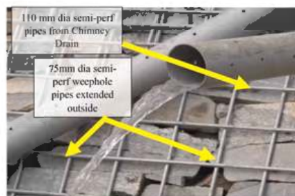
Figure 13. Sub-surface water discharge through weepholes.
