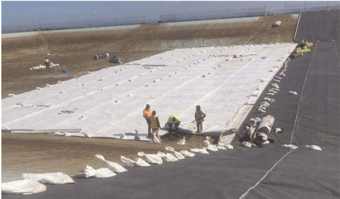
Figure 3. A reservoir with the old discoloured fPP liner being used as a secondary liner. The white material on the floor is a drainage geocomposite and the black material on the slopes and the floor is a conductive non-woven geotextile with a unit mass of about 350 gsm.
