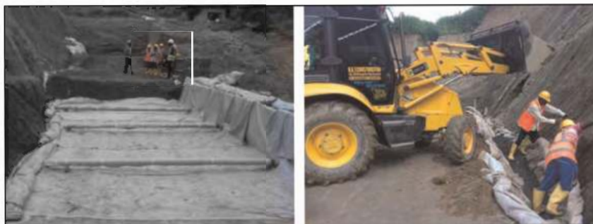
Figure 6. Placement of drainage pipe (left) and drainage blanket at the back of the slope (right).
