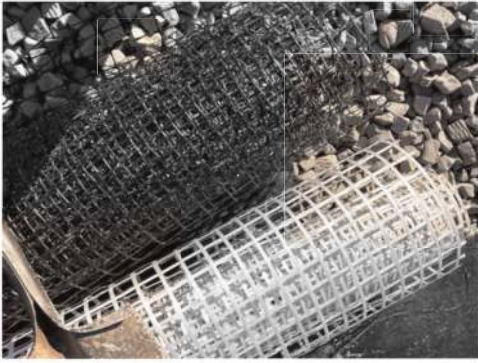
Figure 5. Photo of GS installed at PHL Ron.
