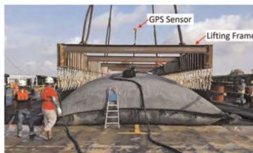
Figure 6. Connecting the lifting frame with geogrid sheet after geotextile tube was fully filled (Geogrid sheet was placed beneath the geotextile tube prior to infilling operation).
