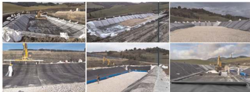
Figure 2. Installation phases of the base reclamation (left to right): 1. Nonwoven and geogrid, 2-3. Aggregate layer, 4-5. Rough bentonite geocomposite, 6. Rough HDPE geomembrane.
