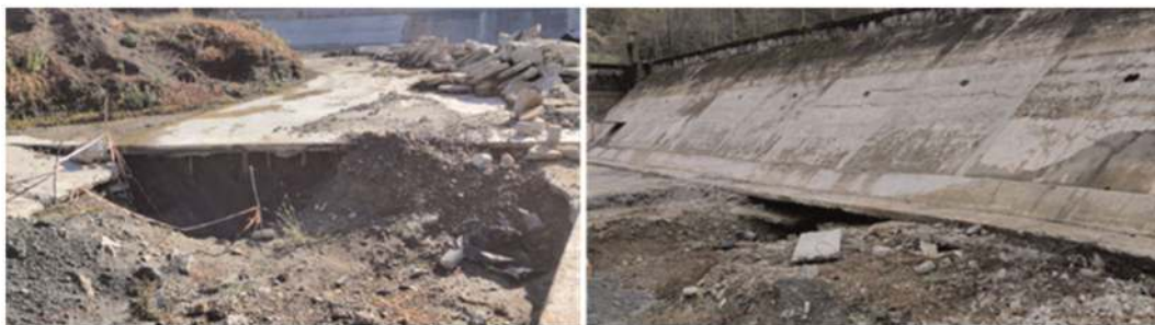
Figure 5. Pictures of the 2020 failure.
