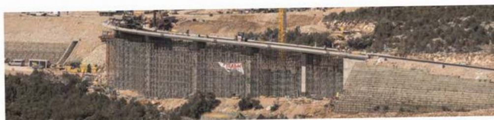
Figure 5. Replacement of external portions of the Brijesta viaduct with reinforced earth embankments (total length about 200 m, maximum height about 15 m).
