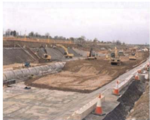
Figure 8b. Membrane over central collector.
