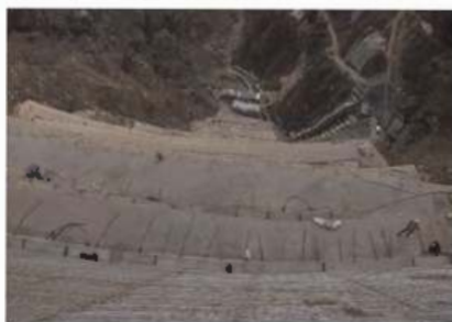
Figure 10. Berm provided to collect & drain surface water.
