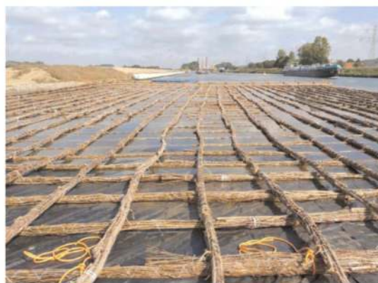
Figure 6. Fascine mattress with geotextile filter layer and brushwood wickerwork as a filter construction underneath ripraps.
