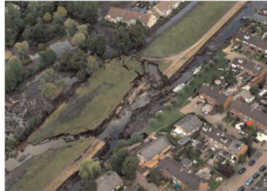
Figure 3. Aerial picture peat levee collapse, caused by dehydration during extreme drought, 2003 Wilnis Netherlands.
