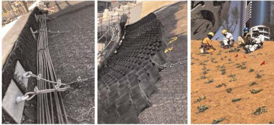
Figure 6. Installation of various geosynthetic components; (a) Macmat HS veneer reinforcement and concrete anchors, (b) Macweb geocell connected through steel cables, (c) Biomac erosion control blanket and vegetation planting.
