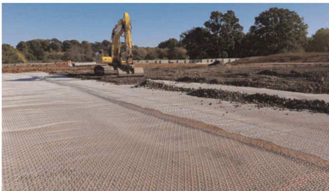
Figure 8. Installation of the working platform at HS2 Stoneleigh Park (Tensar International Ltd).
