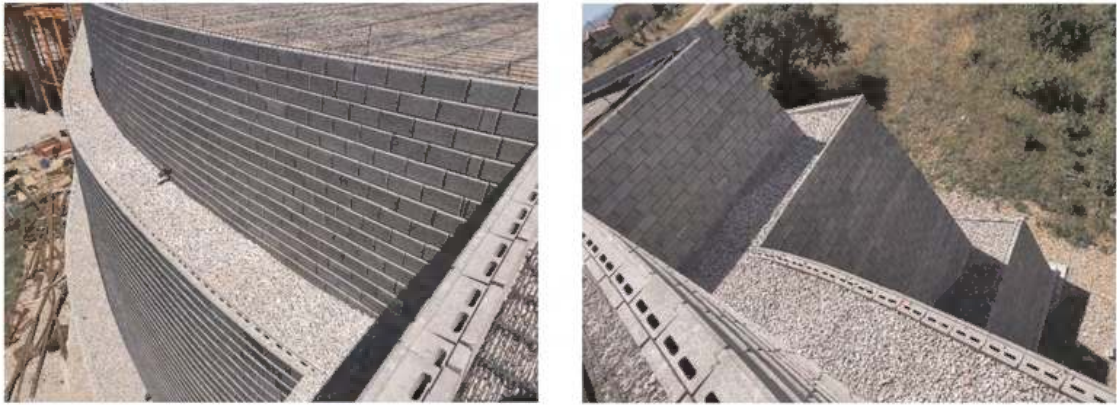
Figure 6. Connection between wing walls and bridge abutments: a) Curved wing wall; b) Angular wing wall.
