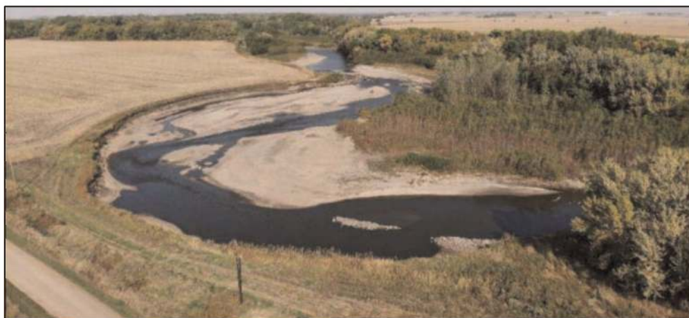
Figure 1. Erosion along West Fork of Des Moines River in 2020 upstream of the Kirby-Flynn bridge.
