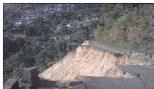
Figure 2. Area where DHR track was totally cut off.
