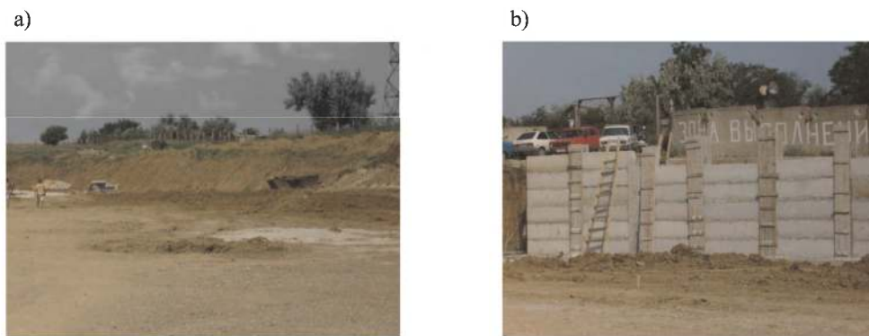
Figure 7. The initial and final stages of the landslide protection structure construction during the 2013 summer in the area of the Vertolit Research Center boathouses location (Prymorske village, Feodosia, Autonomous Republic of Crimea, Ukraine): a) – natural slope: b) undercut slope fixed according to the project. The planned monitoring of the reinforced wall was not carried out due to the annexation of Crimea by the Russian Federation in the spring of 2014.
