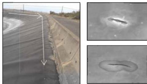
Figure 2. Crest zone of the Buen Paso reservoir, where the geomembrane changes direction and cracks are detected, and examples of cracks.
