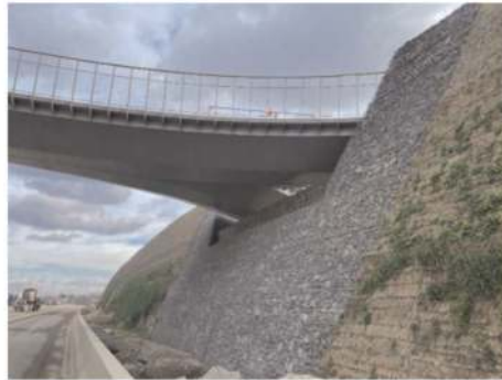
Figure 3. Reinforced soil structure made with Terramesh Green ® and Terramesh Mineral ® units underneath a cycle bridge overpass.
