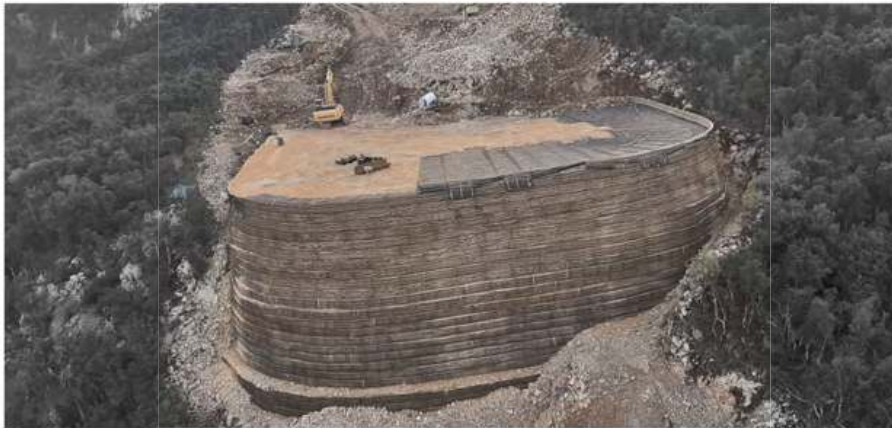
Figure 8. Front drone view of the U4 wing wall and abutment of the Dumanja Jaruga viaduct constructed using a wrap-around reinforced soil technique with a sacrificial steel mesh formwork at the face and mono-oriented extruded geogrids in HDPE.
