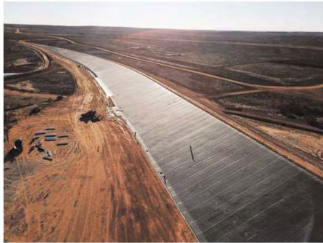
Figure 1. Copper – gold tailings storage facility TSF in South Australia during construction. Note the straight panels on the BGM with no thermally induced wrinkles in extreme 45 deg C heat. This BGM is designed to provide embankment sealing and prevention of tailings migration into sensitive environmental lakes downstream.
