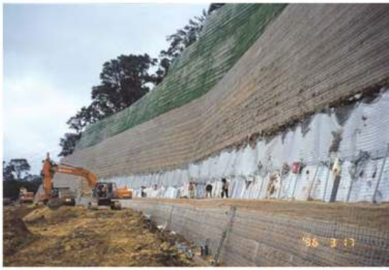
Figure 5. High top-down rock anchored slope with hybrid RSS vegetated slope facing, Taiwan 1996 (AllToffs).
