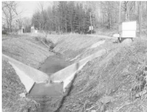
Figure 6. Short-crested V-notch weir replaced the Parshall flume upstream in the view on a larger NAEW watershed.
