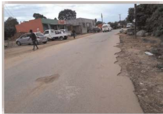
Figure 3. Bangwe to St.Patrick's Road with poor shoulders and without a drainage system.
