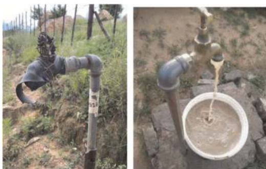
Figure 5. Poorly maintained wate infrastructure.
