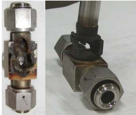
Fig. 5. A burnt valve in a nitrogen trifluoride line caused by adiabatic compression.
