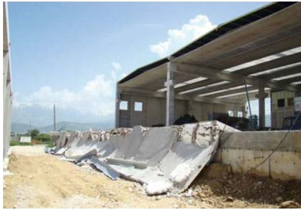
Fig. 4.8 Many cladding panels fell off the structures during recent Italian earthquakes (Toniolo and Colombo 2012)
