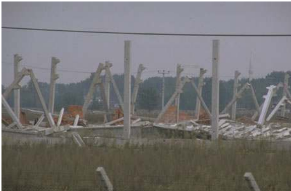
Fig. 4.10 This collapsed precast structure illustrates the importance of ties in precast buildings
