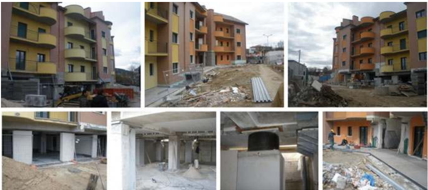
Fig. 14.23 Seismic retrofit of the building complex of Fig. 14.22, performed by means of 42 HDRBs and 62 SDs and connection of the originally separated three buildings. The structural safety will be certified by A. Martelli in 2014
