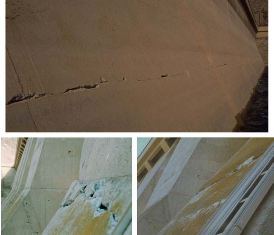
Fig. 20.1 Crack at upstream face ( top ) and at the kink ( left bottom ) and crack showing sliding movement of wedge formed by cracks at the kink ( right bottom ) of the buttress at the downstream face of the Sefid Rud buttress dam caused by ground shaking during the 1990 Manjil earthquake in Iran
