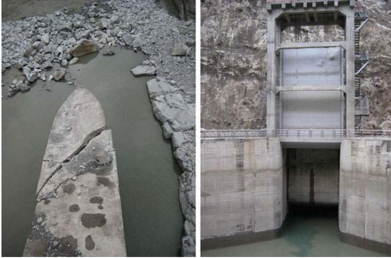
Fig. 20.5 Damaged pier of Futan weir looking downstream ( left ) and damage of sliding gate for power intake (indentation of steel leaf from rockfall) ( right ) caused by the 2008 Wenchuan earthquake in China
