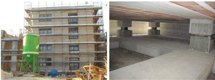
Fig. 14.18 The new block B of the Romita High School for scientific studies in Campobasso (former seismic zone 2), isolated by 12 HDRBs and 10 SDs, which was reconstructed with SI, after its demolition in 2010 (blocks A and B had been found unsafe by ENEA, CESI and the University of Basilicata in 2003 – see Fig. 14.29). The safety of the new building was certified by A. Martelli in 2013
