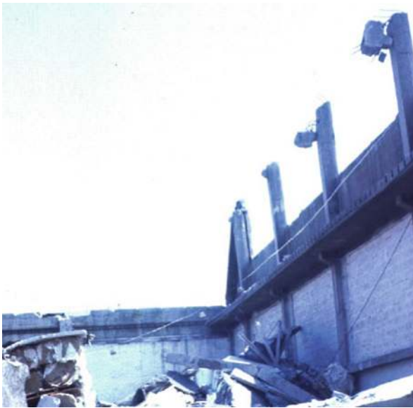
Fig. 4.12 Collapse of the roof system during Montenegro earthquake due to soil effects and poor connections
