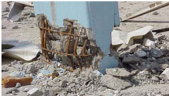
Fig. 4.14 Collapse of a precast column due to poor confinement
