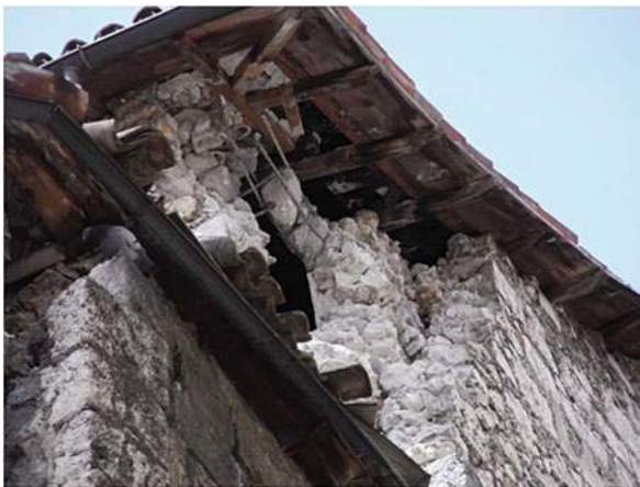
Fig. 15.5 Partial collapse and evidence of a reinforced masonry ring beam in the Church of Santa Giusta in L'Aquila
