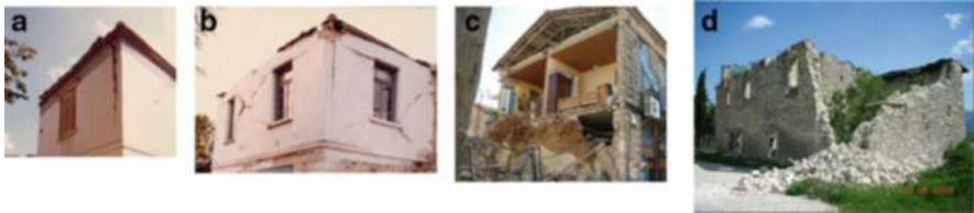
Fig. 8.13 Typical damages due to out-of-plane seismic actions. (a) Typical vertical crack due to out-of-plane bending of the solid wall. (b) Typical vertical crack at mid-length of the wall and separation of walls at the corner of the building. (c) Out-of-plane collapse of wall. (d) Collapse of the corner of a building (due to combined in-and out-of-plane action)
