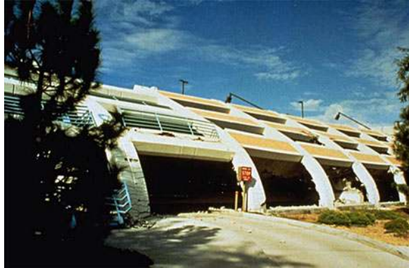
Fig. 1.13 Damage to precast concrete garage structure in the 1994 Northridge earthquake from the EERI photographic dataset for that earthquake (EERI 1995a)
