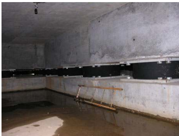
Fig. 14.13 Some of the 193 HDRBs, manufactured in Italy, which protect the building of Fig. 14.12 (picture taken on September 23, 2011, during the 2011 Sochi Conference) (Martelli et al. 2012a)
