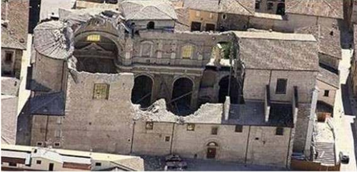
Fig. 15.4 Collapse of the roof and vaults of the church of Santa Maria Paganica, L'Aquila
