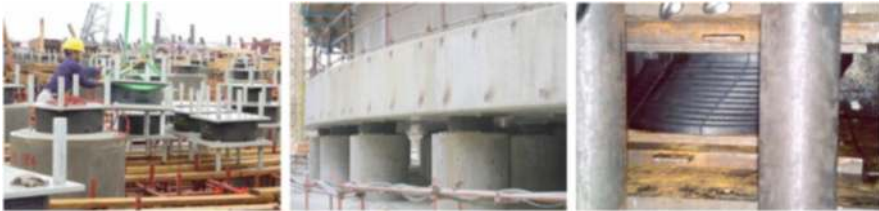
Fig. 14.32 Left : one of the two seismically isolated LNG tanks in the Guangdong Province (Southern China) during construction (each of them was isolated by means of 360 HDRBs). At the centre : some of the isolators after their installation. Right : a HDRB during acceptance tests
