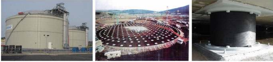
Fig. 14.31 Left : one of the two LNG tanks of Egegaz in Aliaga (Turkey), which were seismically isolated using 112 LRBs and 241 LDRBs. At the centre : view of the isolators during construction. Right : an installed LRB
