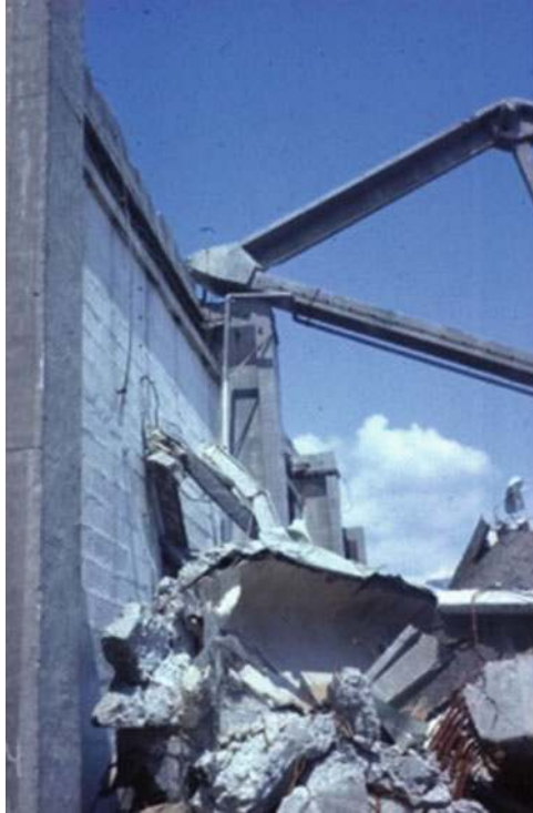
Fig. 4.9 Collapse of the roof structure in Montenegro earthquake due to soil effects and poor connections
