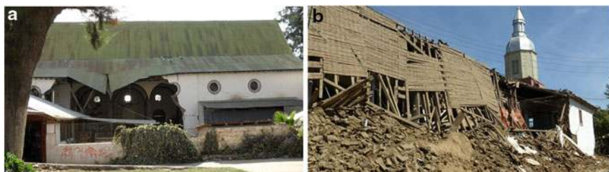
Fig. 15.1 (a) Church in Lalol, Colchagua, Chile. Collapse of the lateral adobe wall, strengthened by shotcrete. (b) Church in Curepto, Maule, Chile. Collapse of the lateral adobe wall, strengthened by shotcrete
