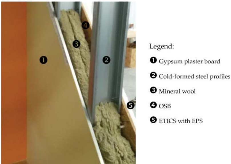
Figure 2. Materials in a LSF wall crosssection [30]. Legend: Gypsum plaster board; Cold-formed steel profiles; Mineral wool; OSB; and ETICS with EPS.
