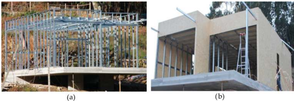
Figure 1. Example of a low-rise LSF residential building at construction stage [14]. (a) Steel frame; (b) OSB external layer.
