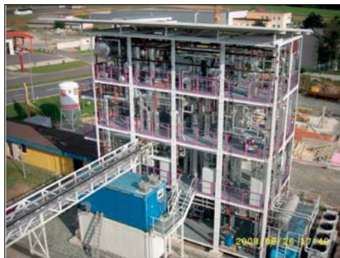
Figure 4. 1 MW capacity SNG demonstration plant [43].
