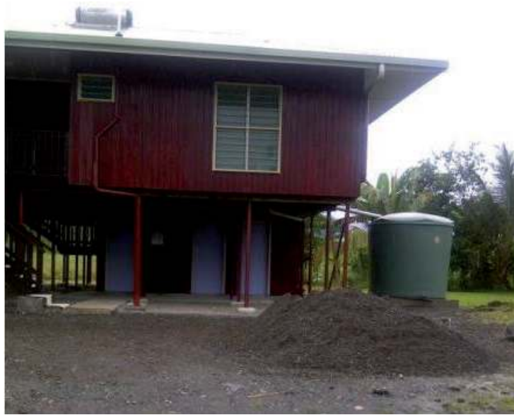
Figure 3. Rainwater harvesting system (RWHS) via rooftop at Papua New Guinea University of Technology. (Adapted from Betasolo and Smith, 2017.)
