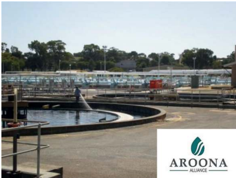
Figure 8. AROONA water infrastructures.
