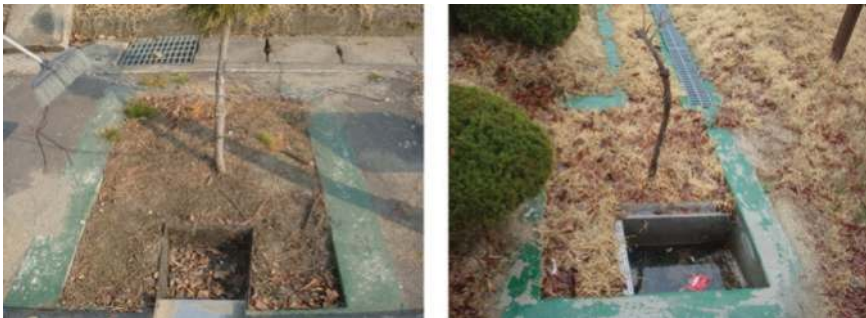
Figure 12.3 Part of the routine maintenance performed in the tree box filter was the inspection of possible accumulation of large debris and litters ( above left ) and checking of standing water and possible clogging ( above right ).
