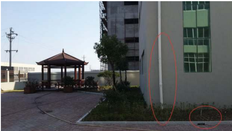
Figure 8.5 Disconnection of roof downspout and rain garden.
