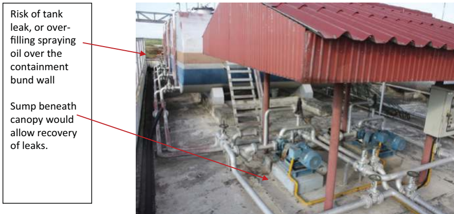
Figure 17.8 Oil storage installation showing inclusion of pump sets within a bunded area, with provision of a canopy to exclude rainfall.
