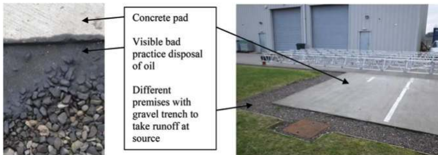
Figure 9.9 Left: Close up of a gravel drain revealing ease of seeing poor practice oil disposal. Right: Filter drains at edge of concrete pad, taking runoff from property in industrial estate, Kinross, Scotland, UK.
