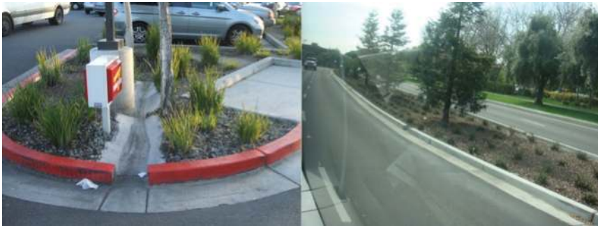
Figure 12.1 Bad design: flow channels were not properly designed so runoff cannot be diverted into the facilities for infiltration (San Francisco/California).
