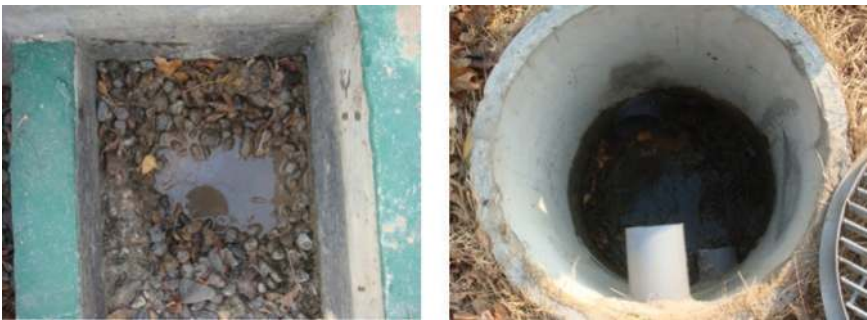
Figure 12.5 Sediment, debris and litter deposition in the sedimentation and facility outlet to drainage access were inspected as part of routine maintenance for the hybrid constructed wetland.
