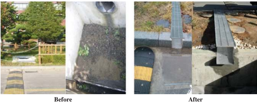
Figure 12.12 The inflow channel of the infiltration trench was renovated as part of the non-routine maintenance.
