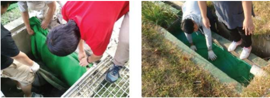
Figure 12.11 As part of the non-routine maintenance, geotextile fabric was replaced in the pretreatment tank of the infiltration trench ( above left ) and hybrid constructed wetland ( above right ).
