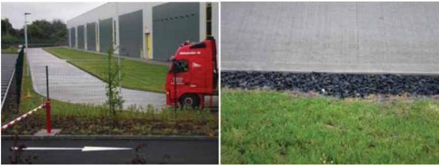
Filter drains at edge of main internal concrete road, taking runoff from truck access route, Dunfermline, Scotland, UK.
