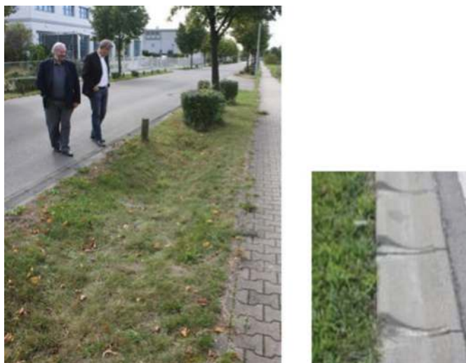
Figure 11.6 Effective drop down kerb line along edge of road, able to feed sheet flow runoff into the under-drained grass swale ( left ) Unfortunately laid line of kerbs on one swale section illustrates risks with good innovations poorly understood by a builder ( right ) Hoppegarten 2014. Photos credit BJ D'Arcy
