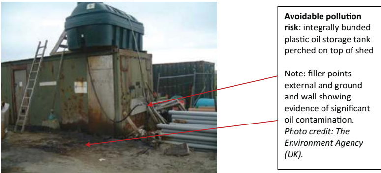
Figure 17.10 An integrally bundled tank that has filler points outside the bund and consequently still presents pollution risks.
