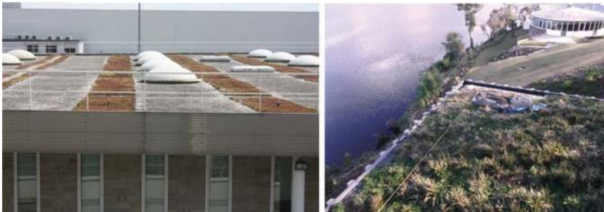
Figure 9.6 Left: Extensive green roof, Charles de Gaul airport. Right: Restoration work on intensive green roof at MONA (Museum of Old and New Art), Hobart, Tasmania.
