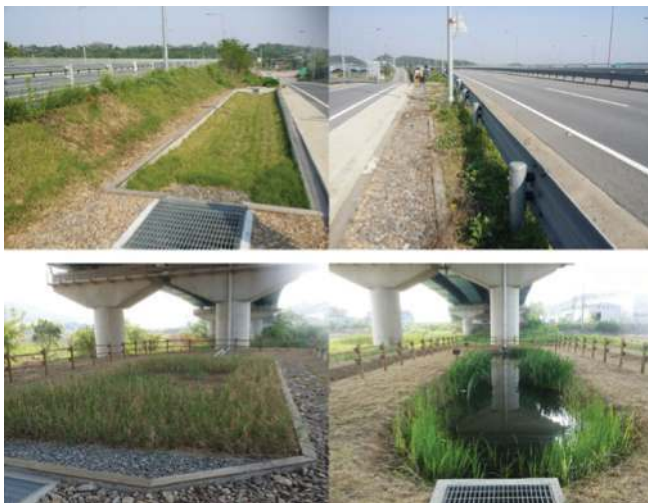
Figure 12.15 On-site photographs of newly-constructed and regularly maintained BMPs in Sejong city, South Korea.
