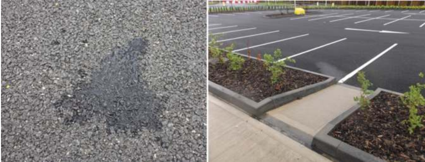
Permeable pavement staff car park (first part of truck access road also drains into this area)
