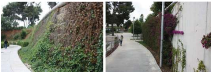
Figure 9.7 Green walls rooted in gravel filter drains, Barcelona, Spain.
