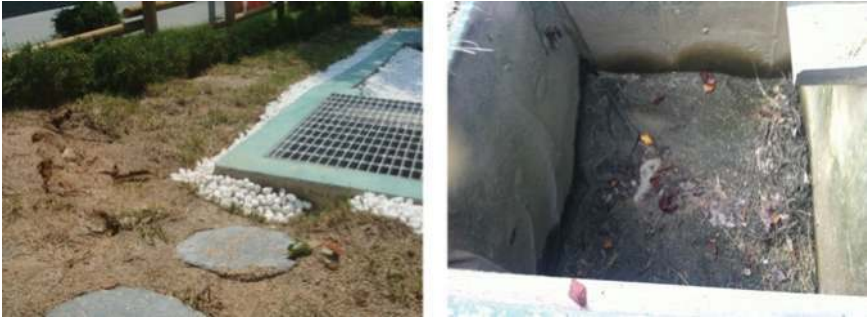
Figure 12.4 Soil settlement ( above left ) and geotextile clogging ( above right ) were also inspected as part of routine maintenance for the infiltration trench.
