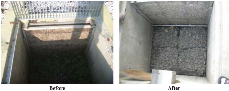
Figure 12.13 Filter media were packed for ease of maintenance in the infiltration trench as part of the non-routine maintenance.
