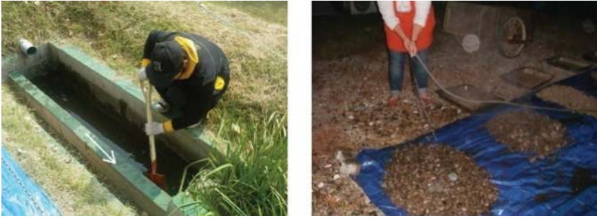
Figure 12.10 Filter media were collected and washed as part of the non-routine maintenance.
