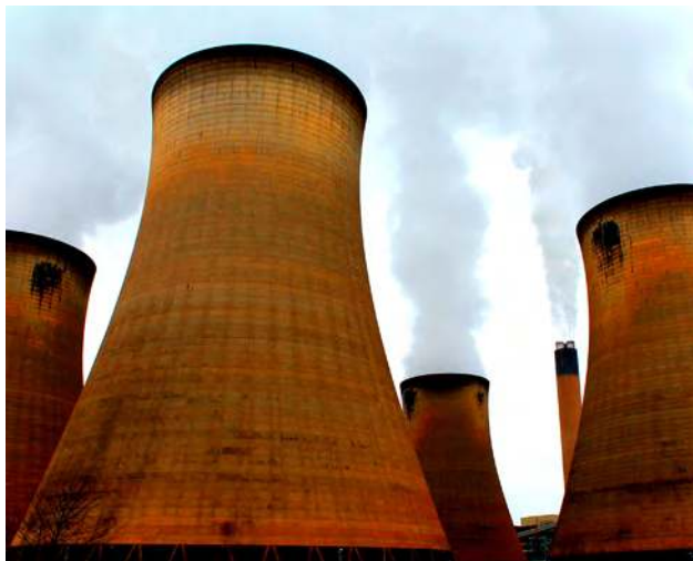
Figure 8.24 Cooling towers at the Drax power station in North Yorkshire, United Kingdom (credit: Les Haines, Flickr)
