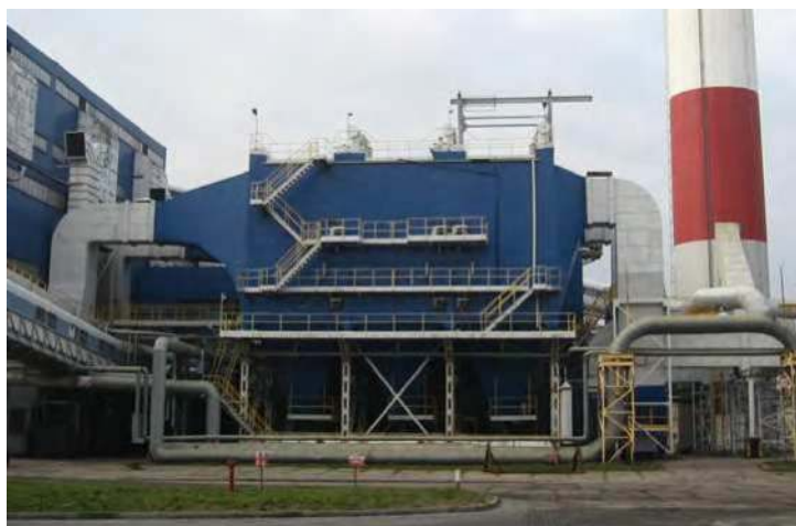
Fig. 1. Electrostatic precipitator in Thermal-Power Station.
