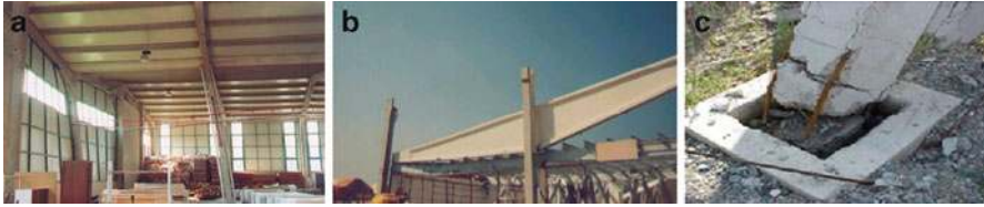
Fig. 8.2 Observed damages. (a) Out of plane deformations of plane frames; (b) Collapse of a rigid roof beam; (c) Plastic hinge at column base
