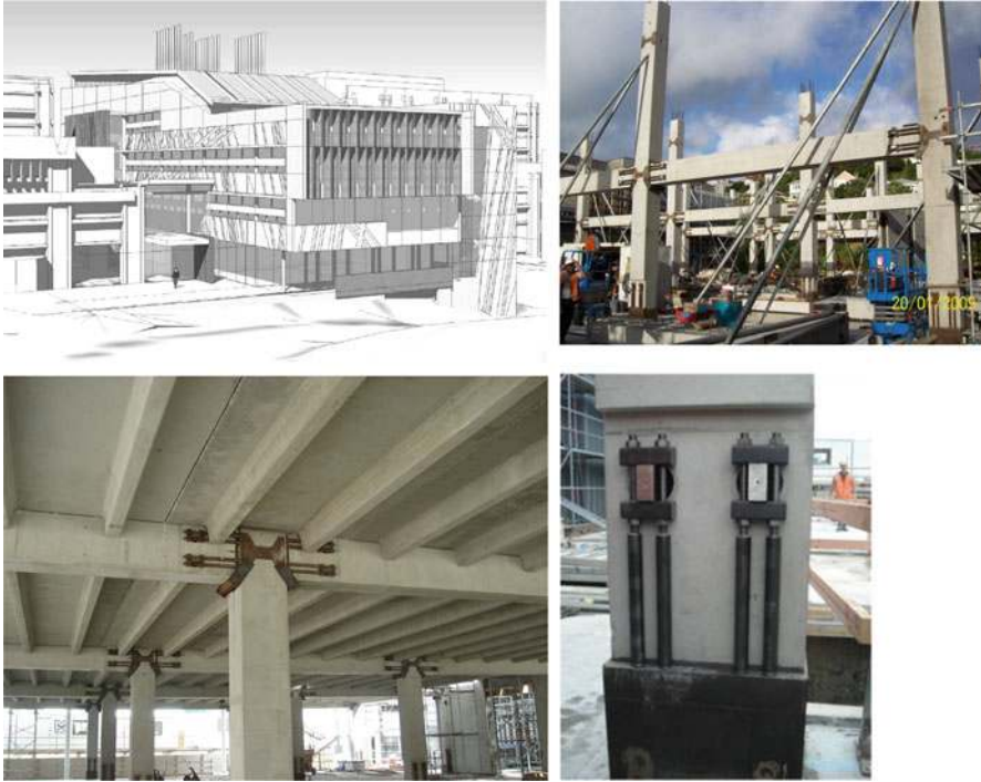
Fig. 13.24 First multi-storey PRESSS-Building in New Zealand (Structural Engineers: Dunning Thornton Consultants; Cattanaich and Pampanin 2008)
