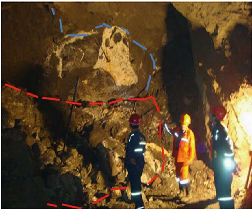
Fig. 9.7 Collapse in 2# tunnel. With kind permission from “PERGAMON-ELSEVIER SCIENCE LTD”: Fig. 5, Wang (2014). All rights reserved
